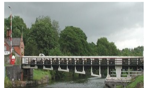
Winnington Bridge- in need of replacement
